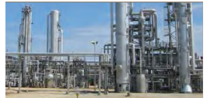
Oil and Gas: use in fuel refineries (DEF STAN 9191), fuel farm, fuel lab and airport fuel transfer
