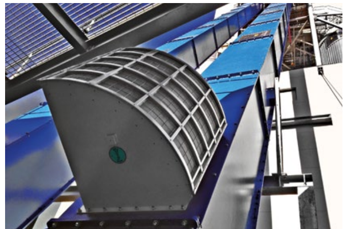
Explosion Safety of a trough chain conveyor using the Q-Box in a biomass power plant.
